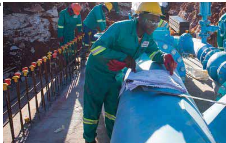
01 As part of the Sishen Western Expansion Project (SWEP) a new water pipeline had been constructed for Sedibeng Water to provide communities with water from the Vaal River some 200km away.
